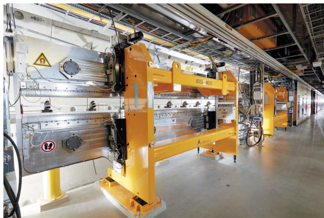
Figure 2 Downstream view along the SASE1 undulator system during installation. The walls for the temperature stabilized enclosure are normally in place and closed as seen in the rear. In the front they are temporally removed for access.
